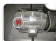
Abnormal Temperature Detection for Motor Overload
