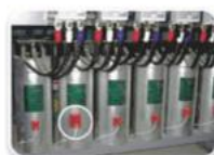
Abnormal Temperature Detection for Capacitor Cabinet
