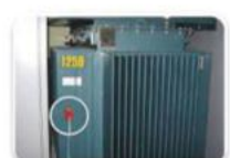
Abnormal Temperature Detection for Transformers
